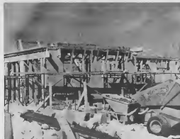
THE TERMINAL building, being constructed by Bohama, takes shape and is ready for the roof raising. Bohama workmen, right, are building the footing that will surround the station. Here they prepare a concrete foundation.
